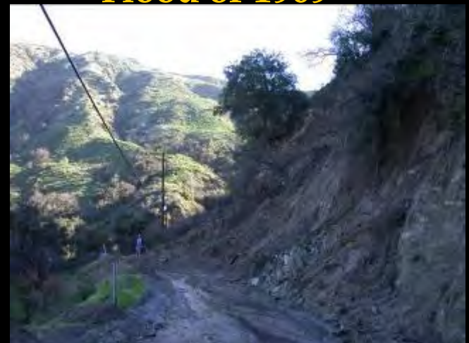
2005 Landslide in San Dimas Canyon
